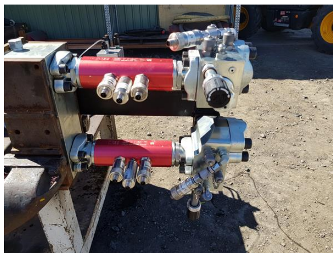
Picture 1: Flow Meter Valves
