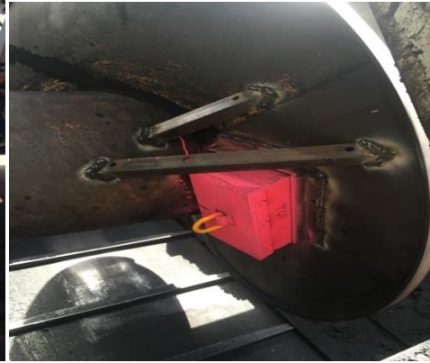
Picture 3 – Gas monitor box on cutter head
