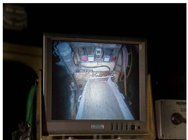
Picture 4 - Close up view of high resolution monitor showing shotcrete discharge into hopper.
