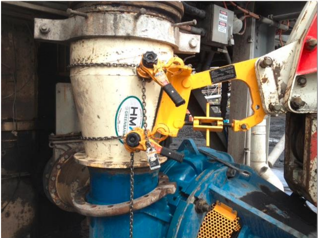
Fig.2 New Acland Coal's Multi-Fit Pipe Lifting Attachment shown in the process of lifting out the discharge spool from a Metso MM-400 Pump. Note there are no Maintenance Personnel located within the potential drop zone.
