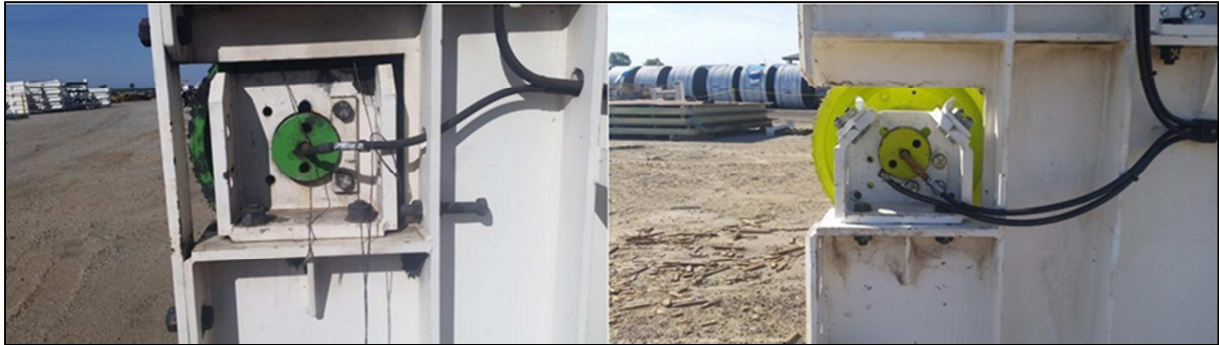
FIGURE 5: Before and after set up on the small diameter pulley in the LTU
