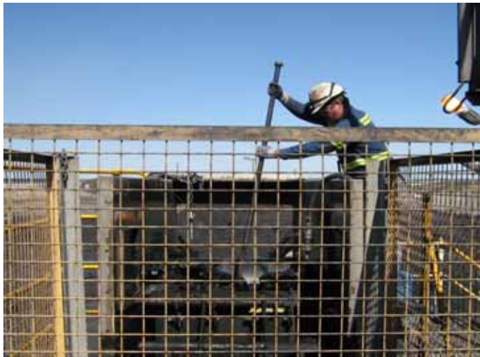
Figure 2: A crow bar being used to assist in the removal of the wedged coal between the deflector plate and the head drum of the conveyor.
