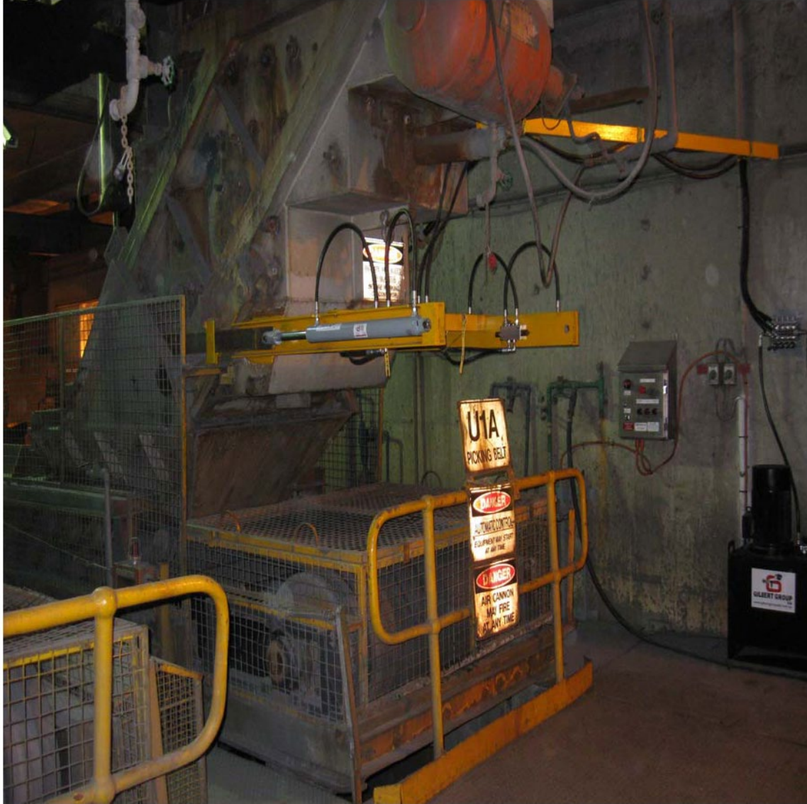
Figure 1: U1A Feeder Swing Chute
