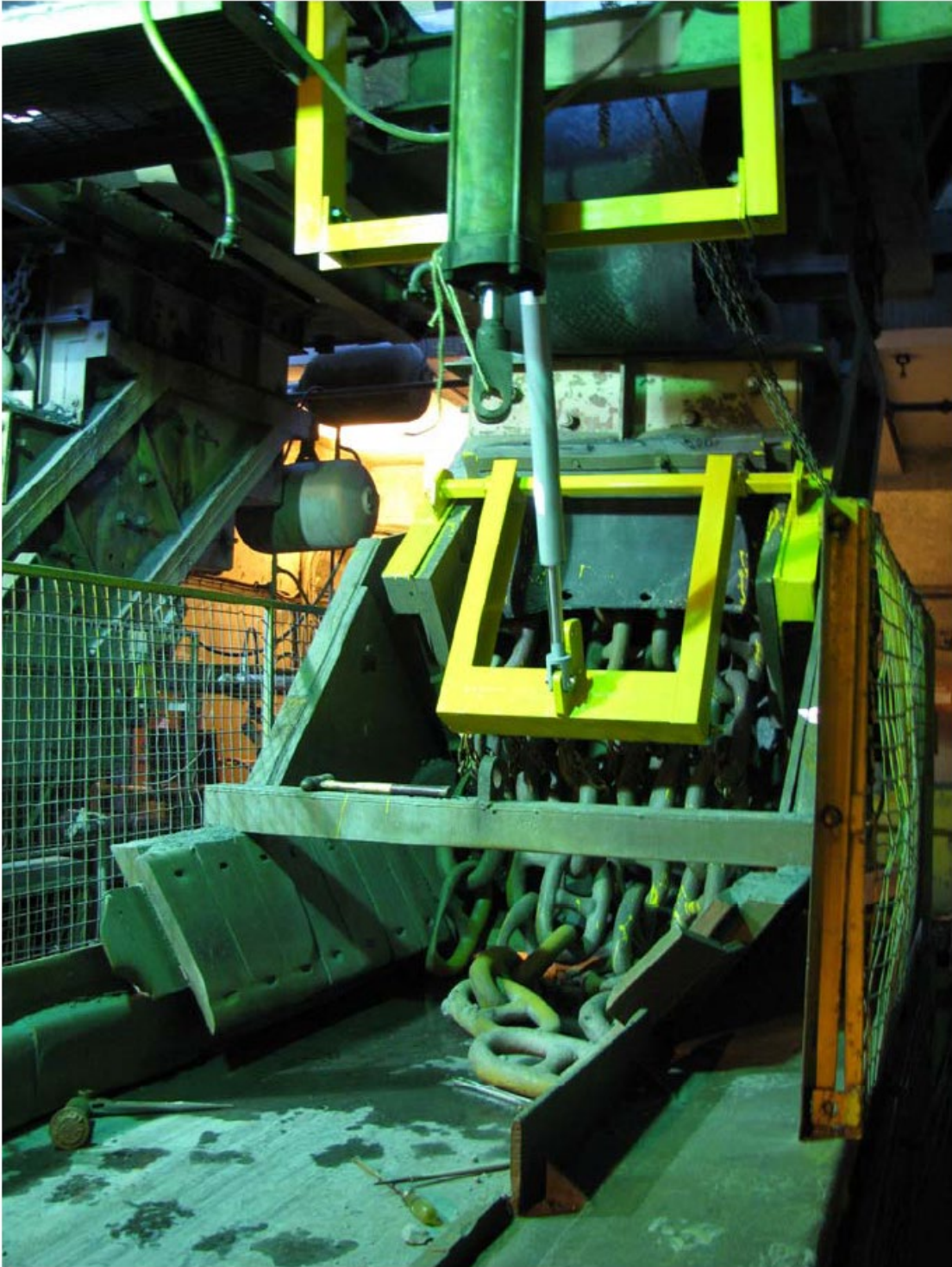
Figure 2: U1B Feeder Chute Room
