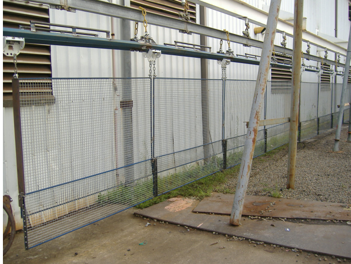
Figure 5 Mock set up of system prior to delivery
