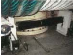
Front of drum. Slack rope roller floating each end on springs with proximity switchers fitted to each end
