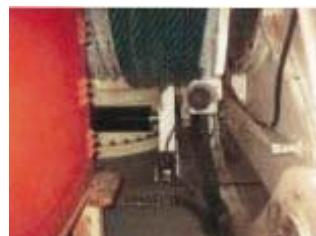
View of the restricted access to the slack rope detector
