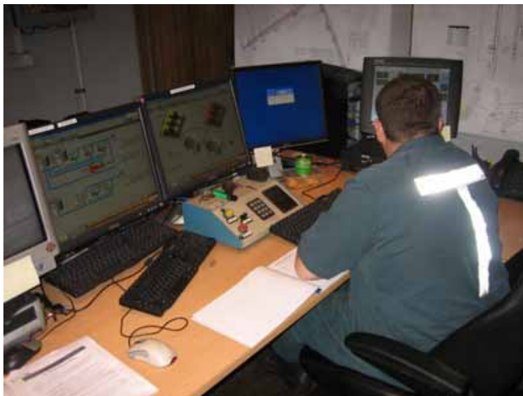
Figure 1. A typical control room.
