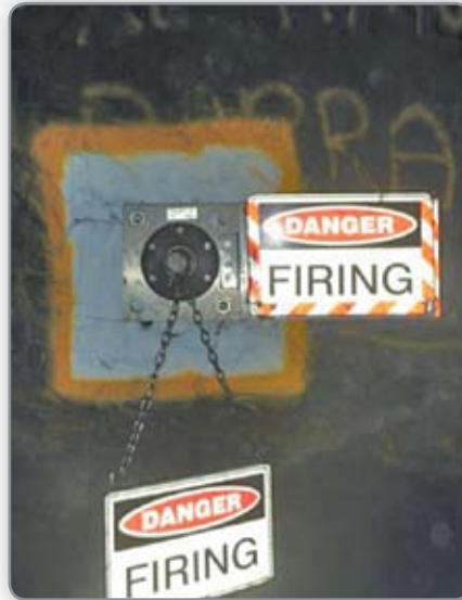
Photo 3: Permanent barricade installed into the sidewall in "closed position"
