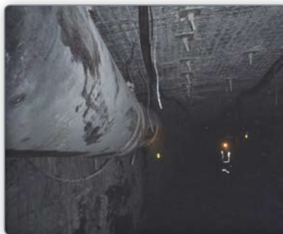
Photo 2: Carbon fibre ventilation tube in production underground mine
