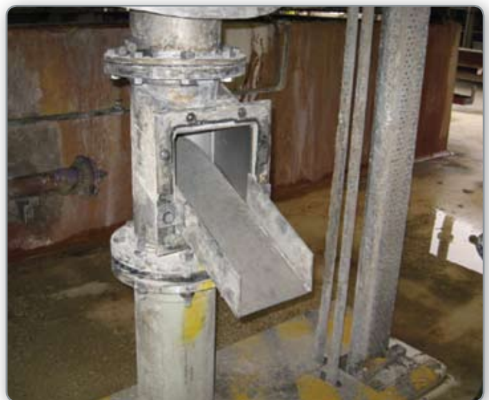
Scale Diverter Chute in place
