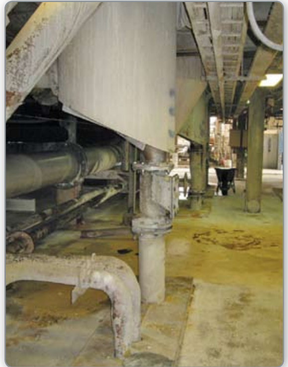
View showing Pipe Assembly at bottom of Filter Vessel
